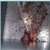
Sludge in tank
